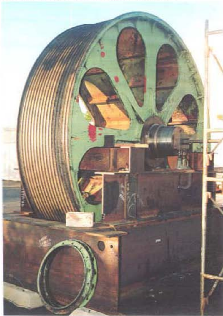
Fig. 2.1 – Counterweight sheave/trunnion assembly in Northbrook, Illinois
