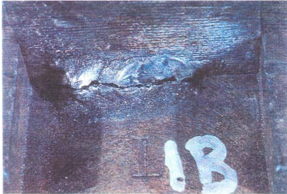
Fig. 2.3 – Cracked key retainer weld at keyway 1B
