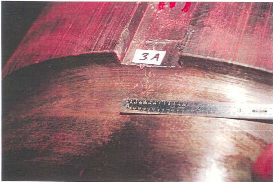
Figure 3 - Surface Discontinuity Detected by MT at Oilway Weld Repair Near Keyway 3A. (Photo Courtesy of WJE)
