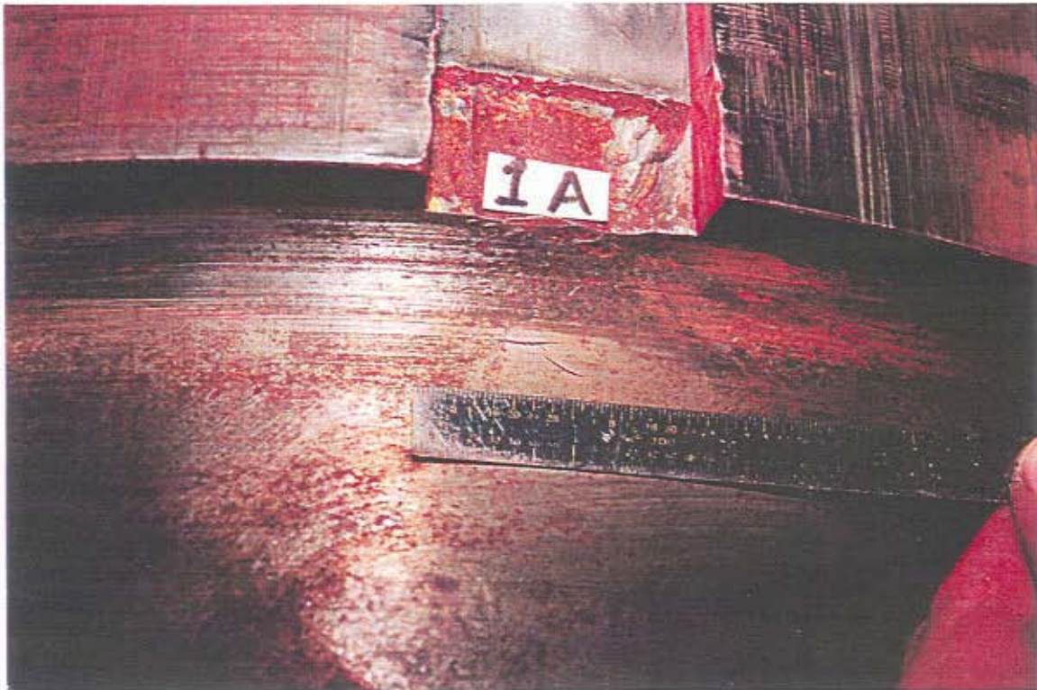
Figure 2 - Surface Discontinuity Detected by MT at Oilway Weld Repair Near Keyway 1A. (Photo Courtesy of WJE)
