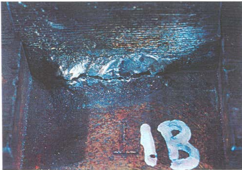
Figure 5 - Typical Key Retainer Fillet Weld Crack Throat Crack (Keyway 1B). (6/99/2-3)
