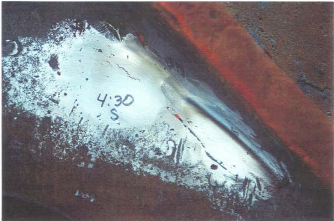
Fig. 3.2 – Apparent shrinkage crack detected in sheave by MT
