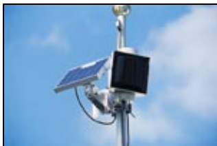
Solar powered transponder reader
