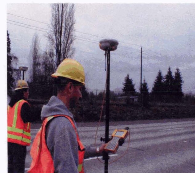
Vancouver Area Engr. Office survey crew using RTK rover receivers for location survey
