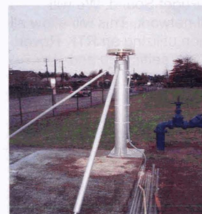
Puget Reference Station Network (PRSN) base receiver
