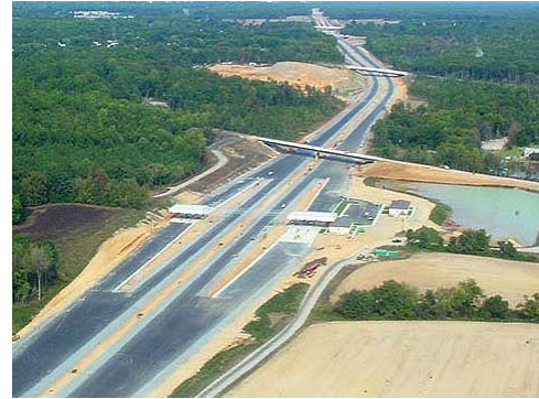
New Toll Plaza with Lanes Split for ETC and Manual Toll Collection
