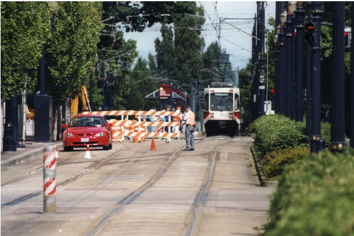
Photo: Single track operation at emergency cross-over on the MAX Blue Line
