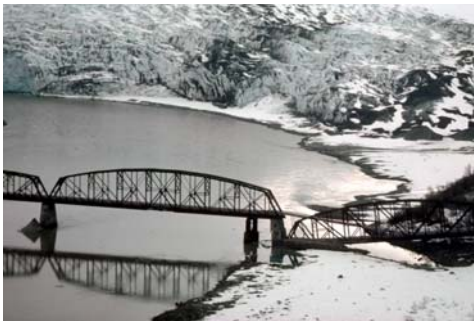
A span of the "Million Dollar Bridge" in Alaska slipped off its foundation during an earthquake in 1964.
