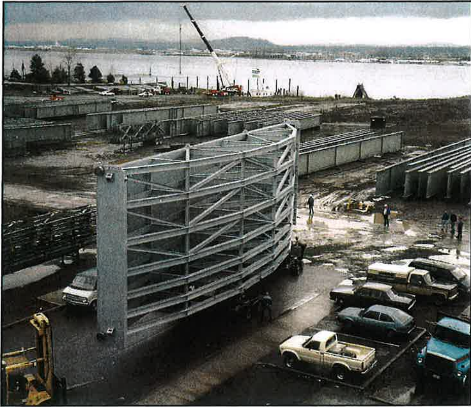
Up-Stream Navigational Lock Gate (1991)
