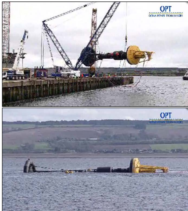
Figure 9. 150 kW Wave Energy Buoy by OPT, 140 feet long, 40 feet wide deployed
